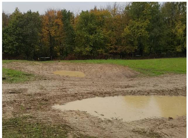
Figure 4. Sunken land drains (top-left), excavated land drains (top-right) and a series of scrapes to intercept the drains and overland flow paths
