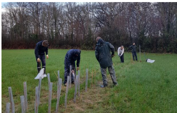
Figure 4. Excavator cutting through river embankments to increase washland inundation (top), volunteers planting a cross-slope hedgerow (bottom)
