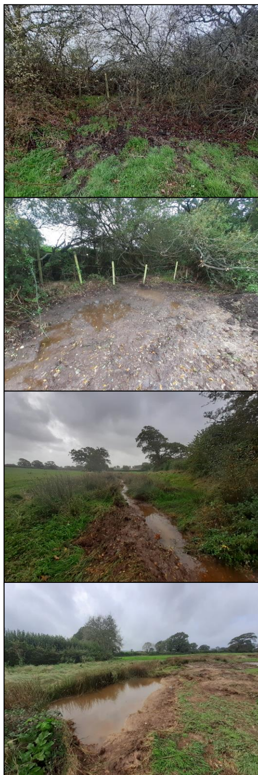
Figure 3: Through creating a cutting through the bank disconnecting the ditch from the old stream channel (Top), we have reconnected the stream and enable high flows to enter it and spill out across the floodplain. We created four new four online ponds (Bottom), as well desilting an existing one.
