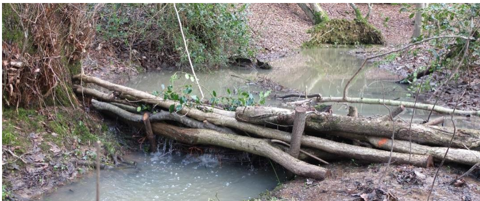
Figure 1. Leaky dam constructed to allow low flows to flow unimpeded, but to intercept, slow and divert flood waters
